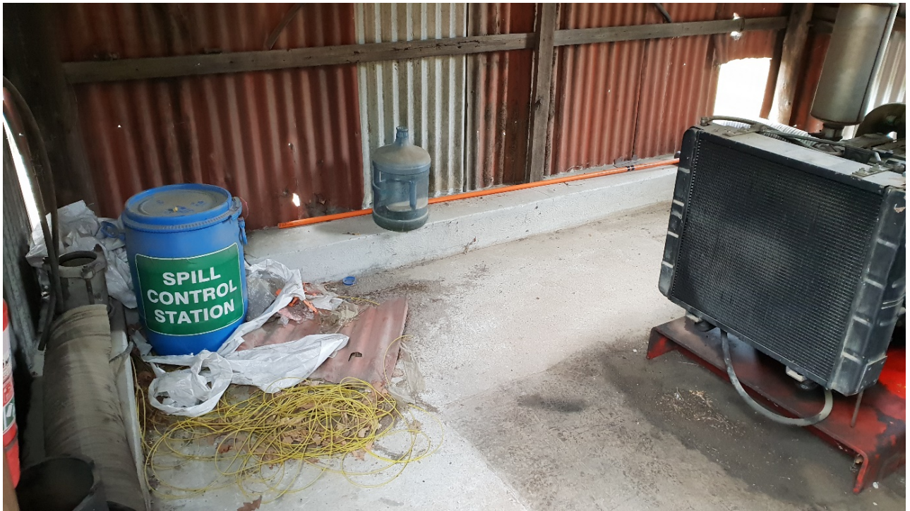
Photograph 15: Spill kit in pump shed at Donazzans Dam.
