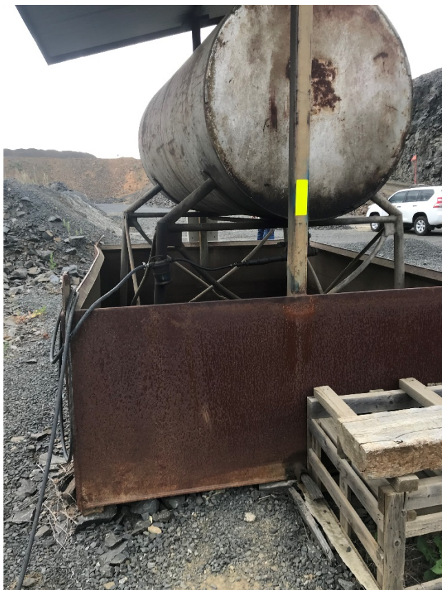
Photograph 9: Diesel tank at quarry pit – bund drain pipe is open.
