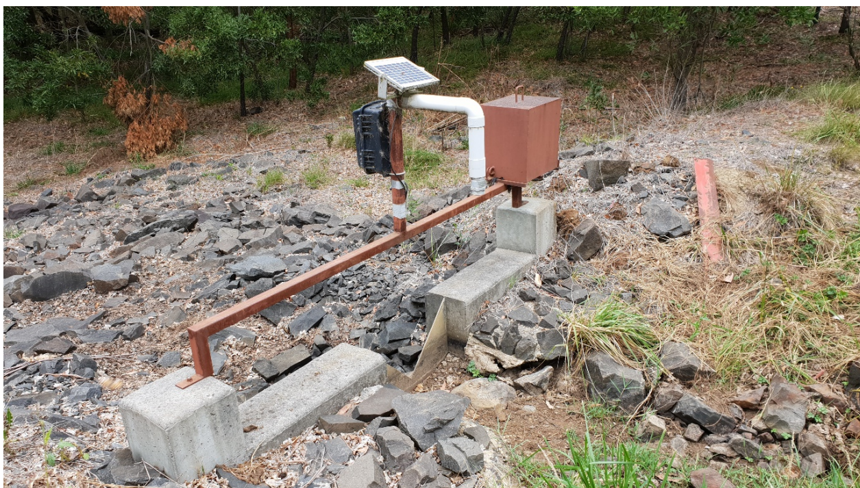
Photograph 17: V-notch weir at EPA sampling point. Bare earth above sampling point could affect turbidity of discharge; soil should be stabilised here.
