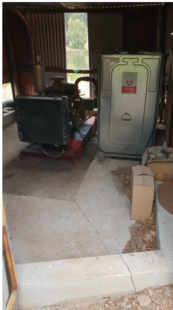
Photograph 16: As above – bund is cracked however fuel tank is double-skinned.
